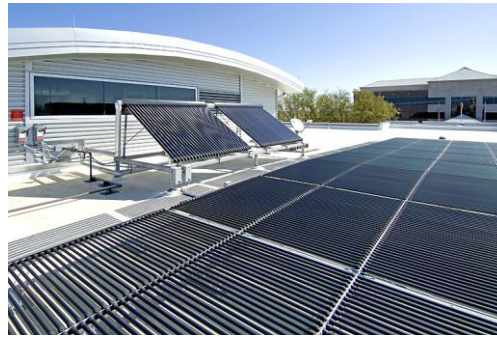
Roof mounted photo voltaic solar collectors generate electrical power
